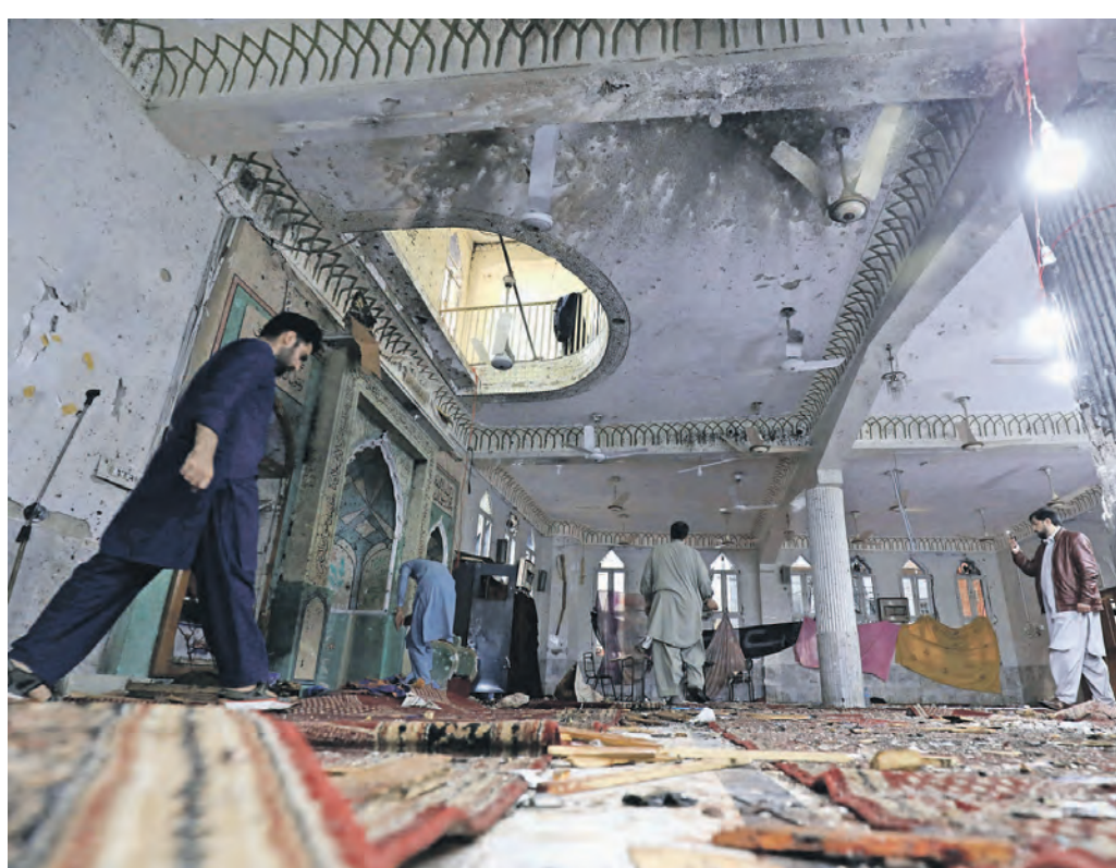
Investigators survey damage at the Kucha Risaldar Shia Mosque's prayer hall in Peshawar, Pakistan, after a suicide bomber attacked Friday with a crude, ball-bearing-laden device. FAYAZ AZIZ/REUTERS
